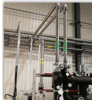
● Oil and Cooling water for Machinery.
