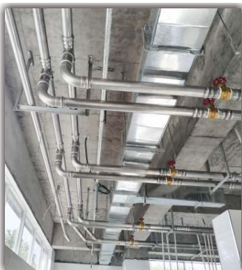
● Cooling water for IT industry.
